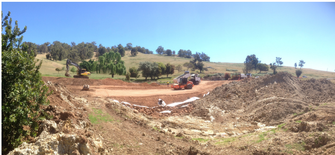
Tweed Road Failure and Corrective Works
